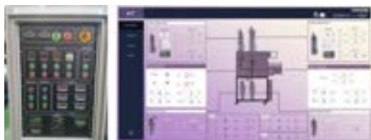
Figure 10. Control Panel and monitoring system
