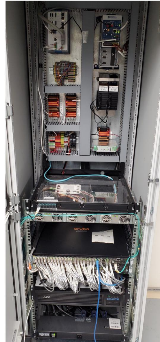
Fig 2. Main Industrial Control Enclosure
