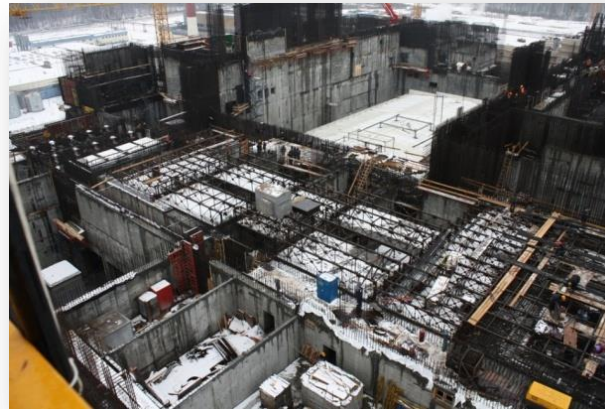
Steam Generator Compartment of Main Building
