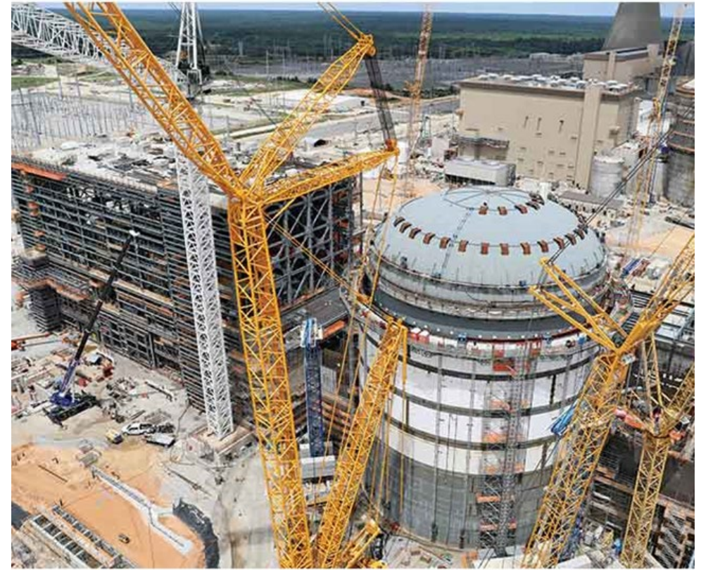
Containment dome at plant Vogtle under construction. Vogtle is an LWR type plant.
