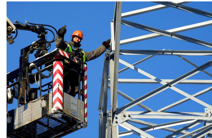
Construction of electricity transmission lines began: installation of supports and installation of wires (end of December 2023)
